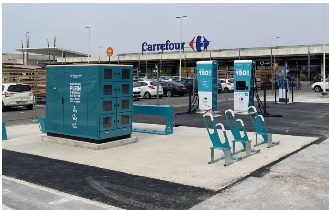
Photo of the station being built at the La Chapelle Saint Luc – Troyes hypermarket
